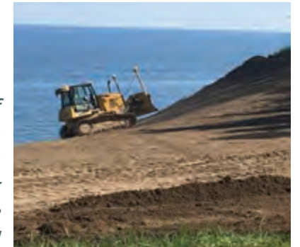
Bluff stabilization in progress in August 2022 by Bill Debus of the News-Herald
