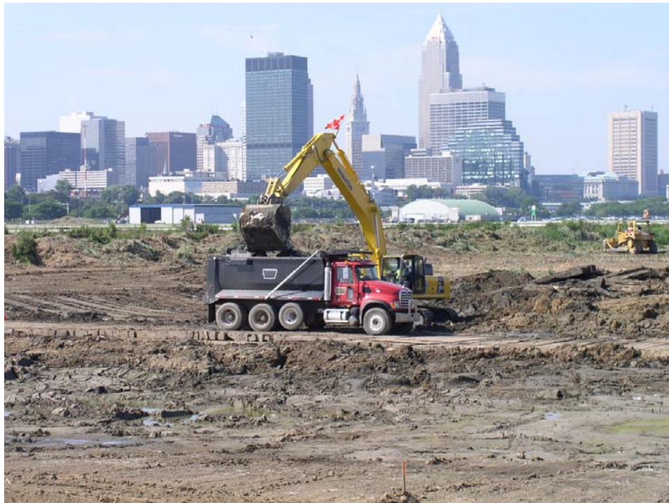
Figure 2-1. Excavation in 2010 at existing CDF 10B for re-use at the Cuyahoga Valley Industrial Center.
