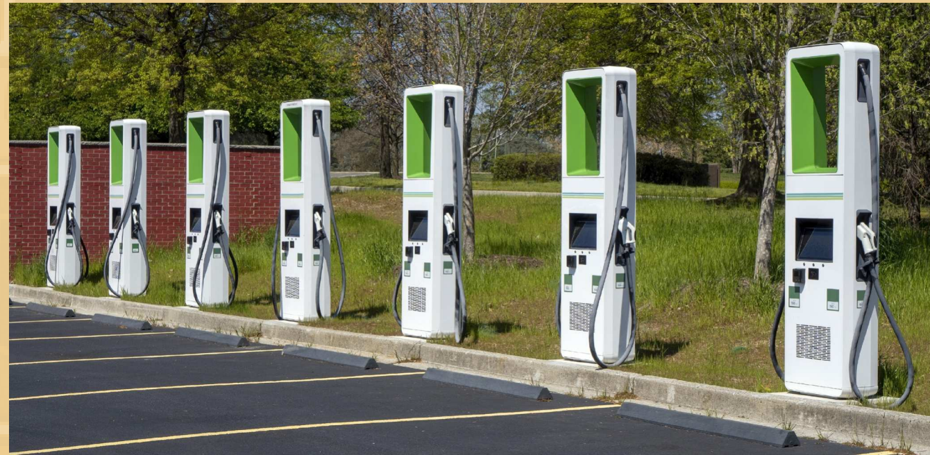
Figure 6-30. Electric Vehicle Charging Station
